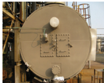
Incinerator after HPC® Coating application was 122°F (50°C).
