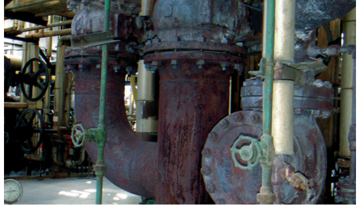
Pipe system before HPC® Coating application, showing extensive CUI
