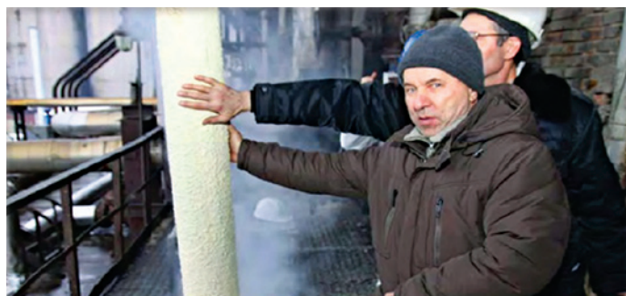
This pipe surface was 872°F (467°C) before coating. These men were able to touch the pipe after only 25mm (1") of HPC® Coating was applied. Additional coating thickness was added to complete the project for long-term performance and durability.
