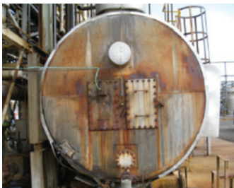
Incinerator before HPC® Coating application was 356°F (180°C).
